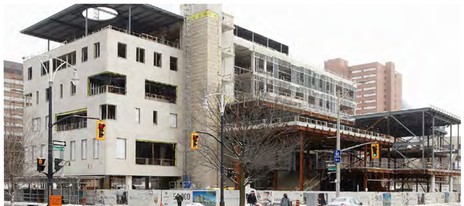
▲ The southwest view of construction of the McMaster Health Campus in downtown Hamilton.
